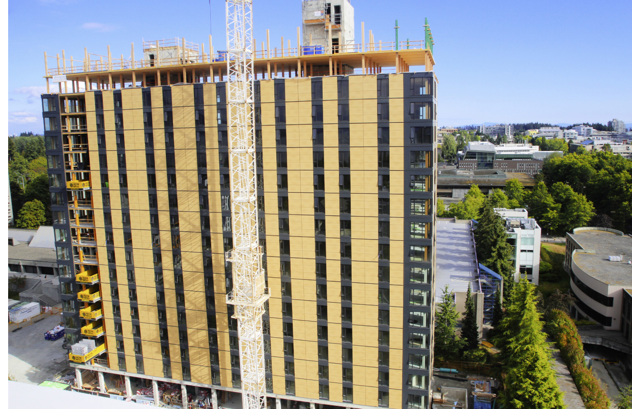
Brock Commons student residence in Vancouver, Canada, by Acton Ostry. Photos Acton Ostry Architects Inc. and University of British Columbia
